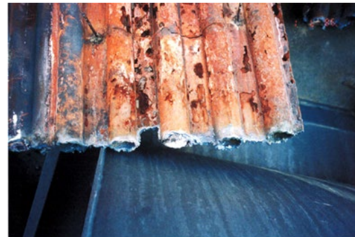
The surface crack along these tubes is a result of severe overfiring.
